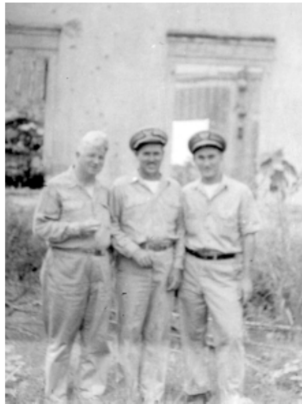
A building used by the Japanese headquarters received a direct hit by a 500-lb. bomb
